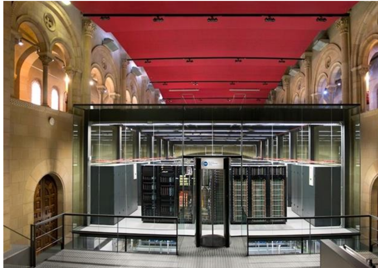
Marenostrum, (Barcelona Supercomputing Center)
